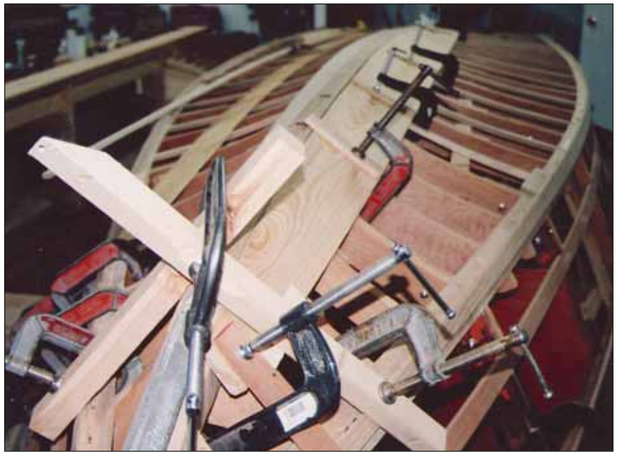
There's no such thing as a square corner on a boat, something these multiple clamps attest to. After 72 years of service, MAB needed to have nearly all its wood below the waterline replaced.
